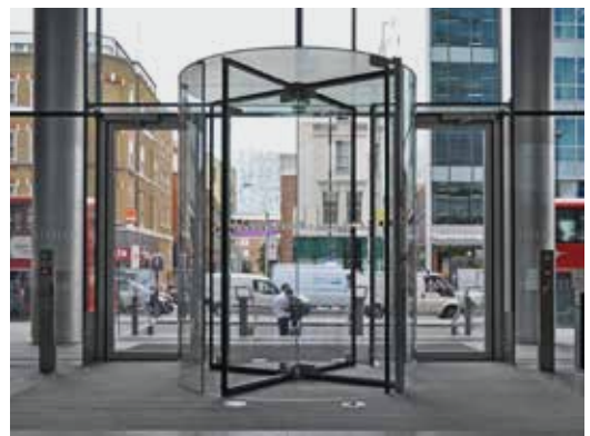
Power operated revolving door
