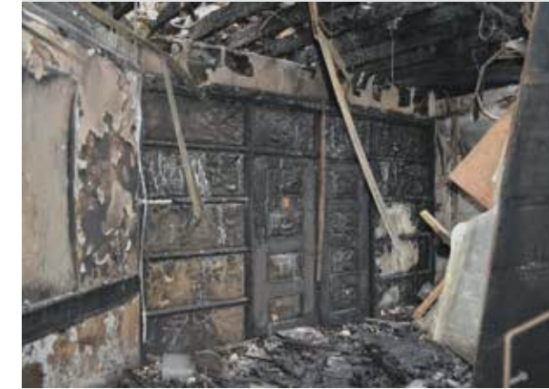
Internal side of fire door after fire
